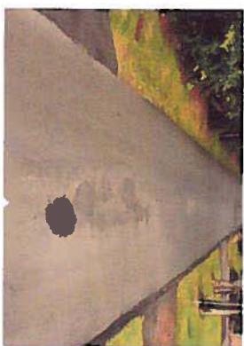
Halekou Road PCI Category: Poor
