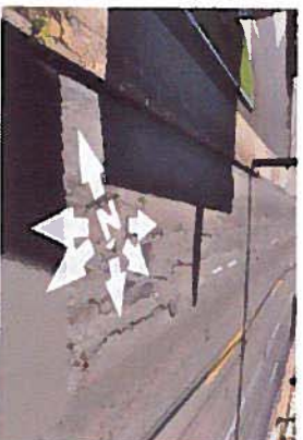
Waiatae Avenue PCI Category: Failed
